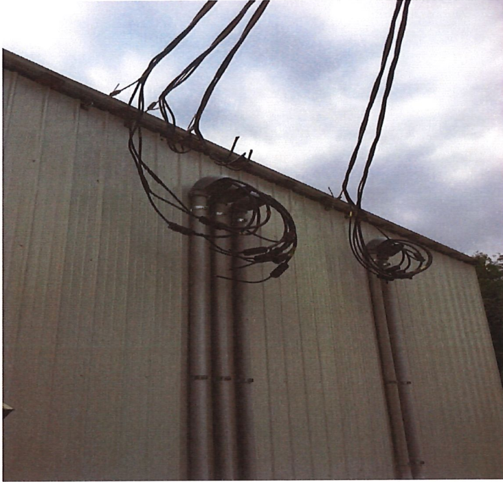
T1 Service Conductors
