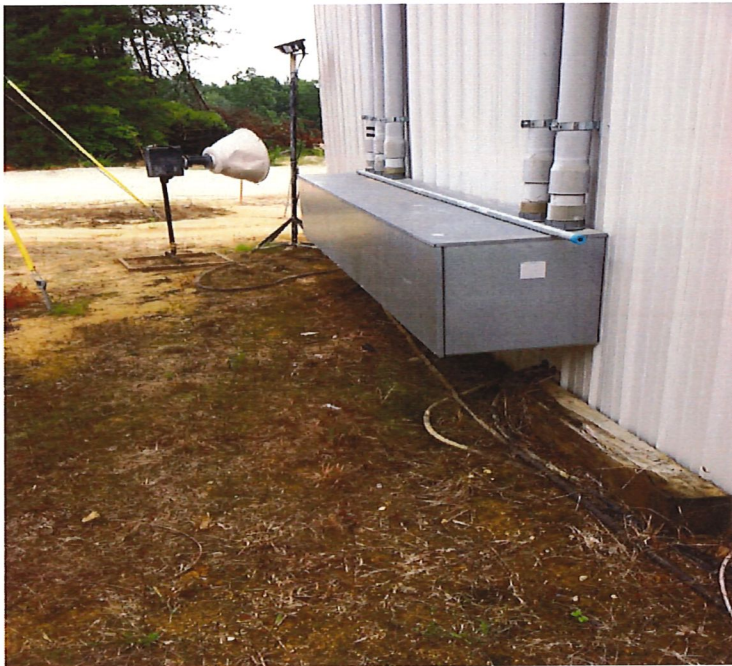
T1 Service Wire Way and Grounding Trough
