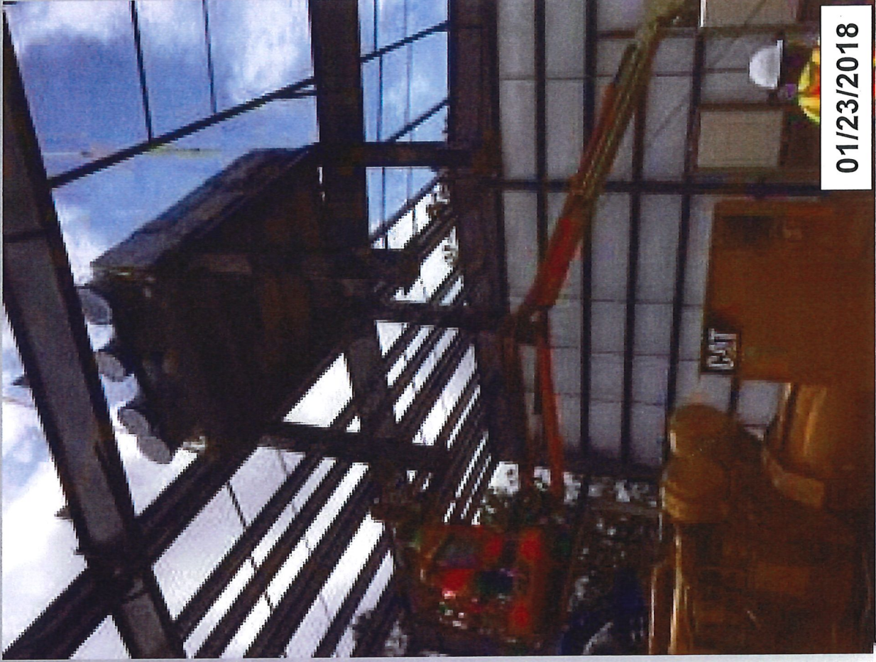
Placement of clean emissions module just prior to putting roof on building
