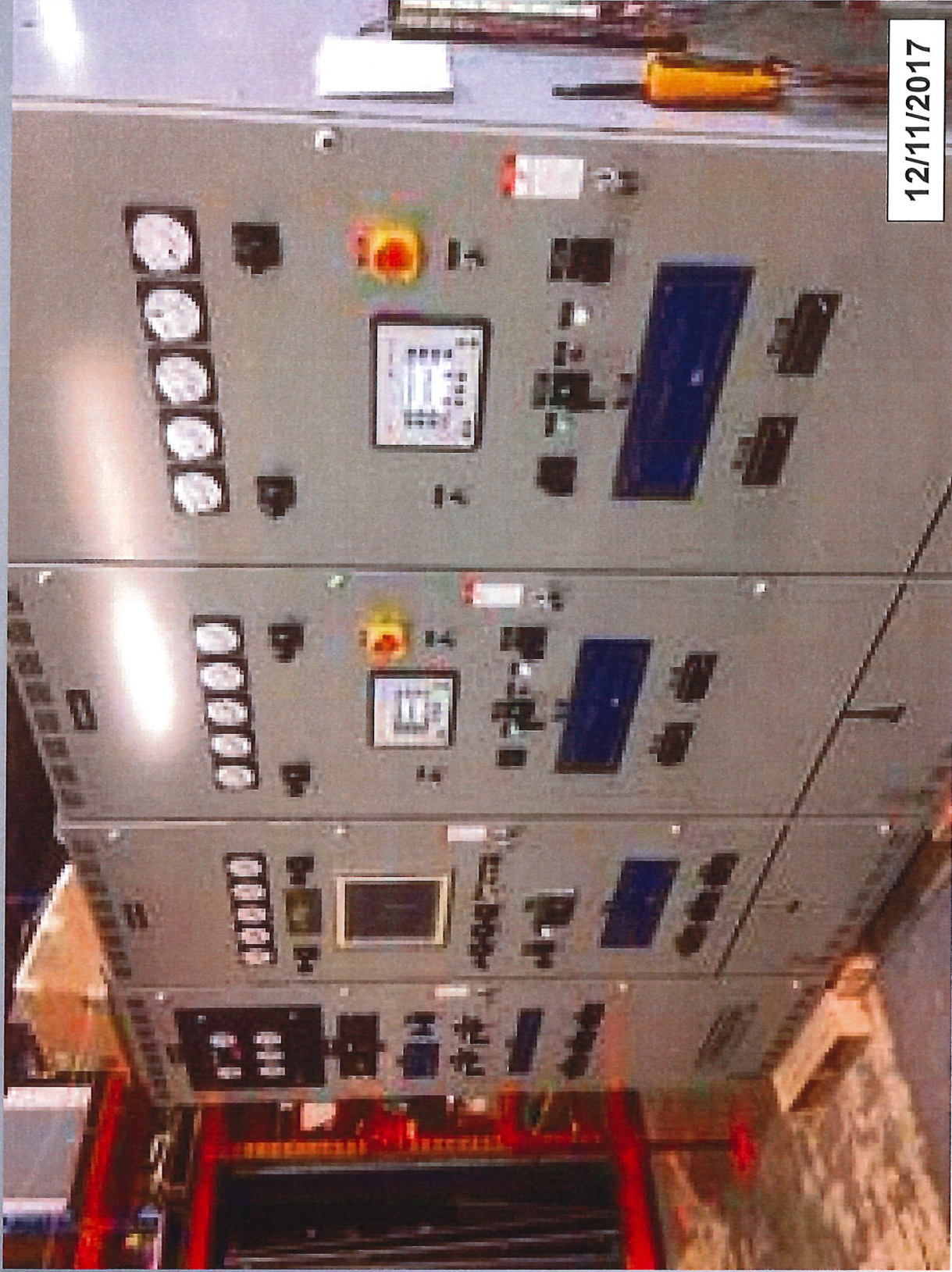
Control and switchgear as it sat in Thompson Electric Shop in Vancouver during factory acceptance testing witnessed by Georgetown, UTEC and Blanchard Staff
