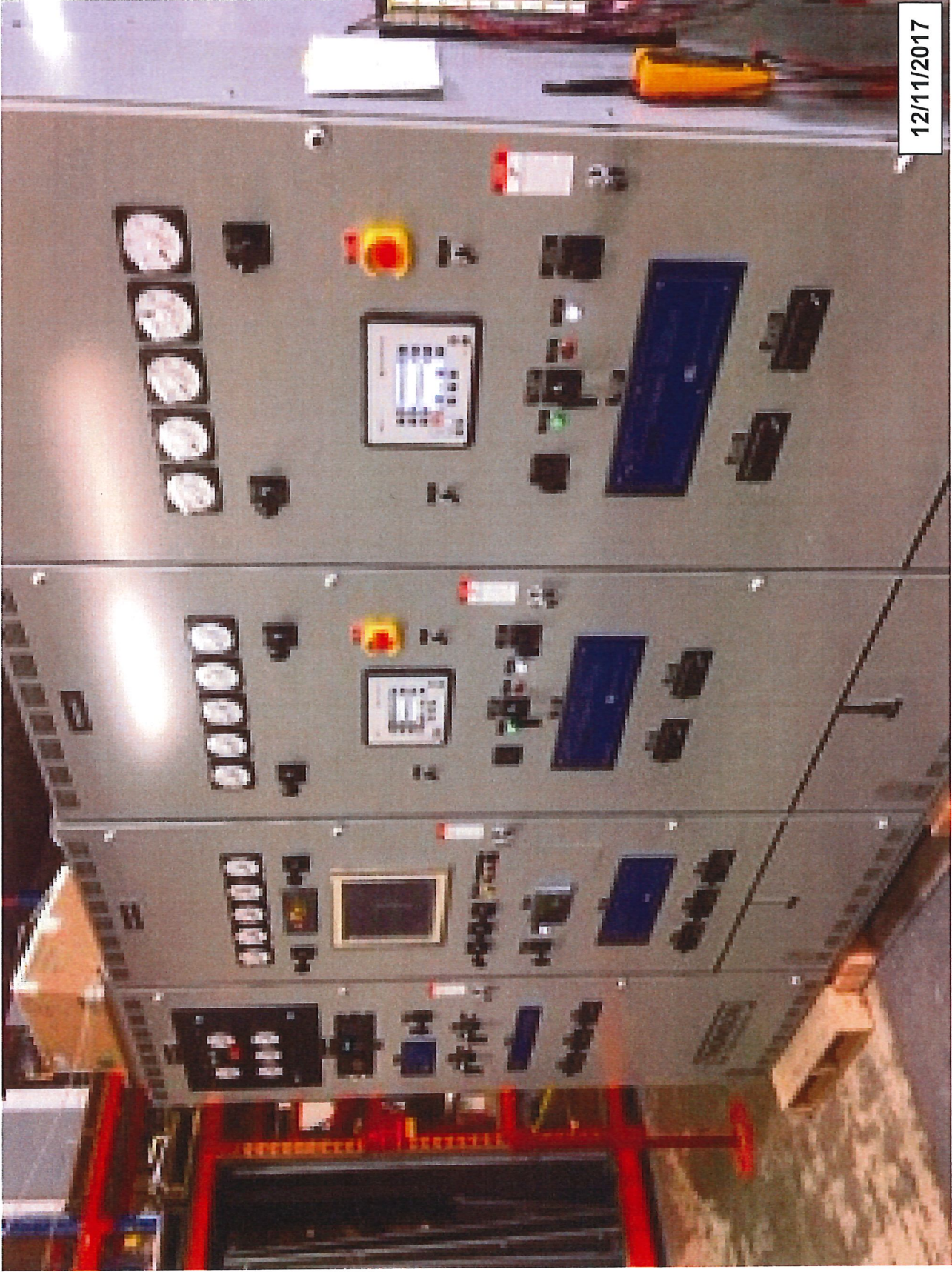
Control and switchgear as it sat in Thompson Electric Shop in Vancouver during factory acceptance testing witnessed by Georgetown, UTEC and Blanchard Staff
