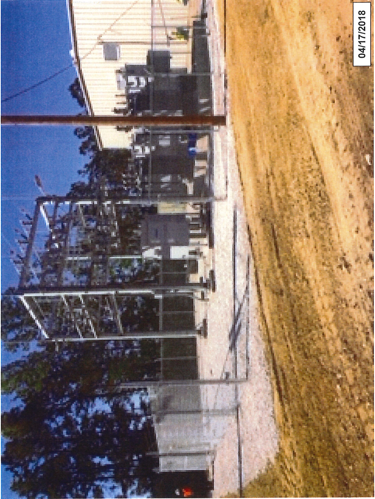
Substation finished and fenced. Breakers required for switching to provide automatic emergency backup for waste water treatment plant
